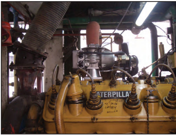
■ The EGC 4 is mounted on a Caterpillar 3408 gas compressor in India.
