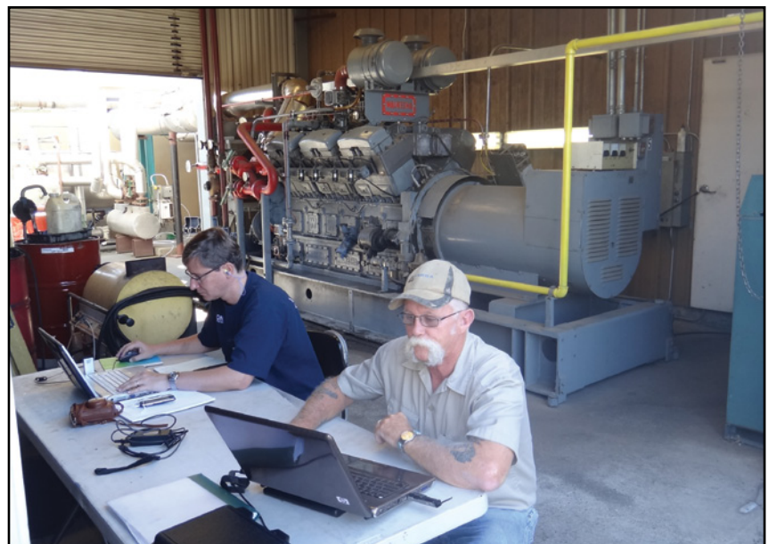
David Campbell of Continental Controls and John Vronay of Vronay Engineering monitor the operation of the engine via their computers.
