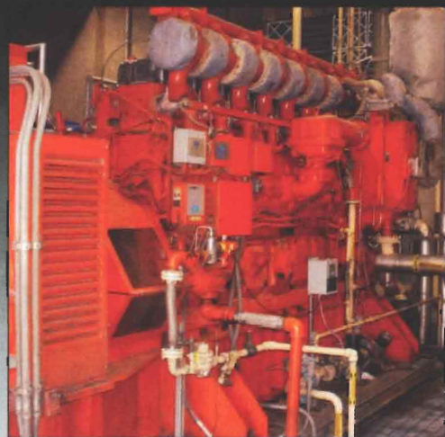
Lean Burn Application – 8 Cylinder Waukesha AT running on 500BTU digester gas. Photo courtesy of Continental Controls.
